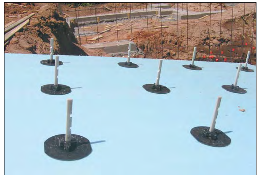
A close-up of the rigid form insulation and unique tie system used to suspend the insulation between the forms.
